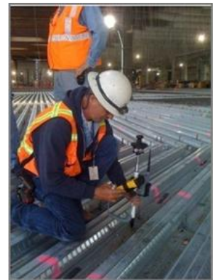
One person can accurately lay out hundreds of points in a single day.
