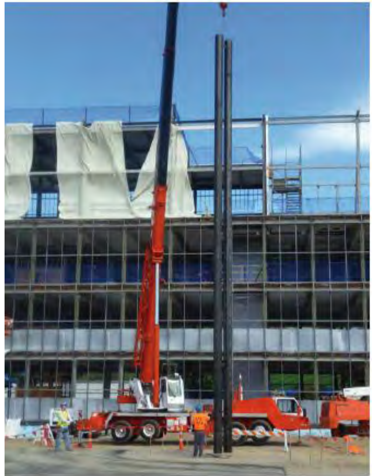
Mechanical components can be prefabricated and shipped to the job on flat bed tractor trailers and installed with cranes, thereby reducing field time and exposure to hazardous work conditions around open shafts.
